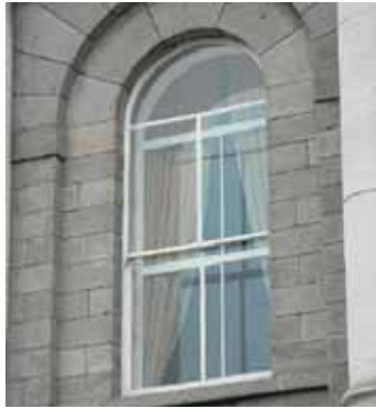
Unsympathetic plastic exterior glazing installed on an historic property in Dublin, Ireland
